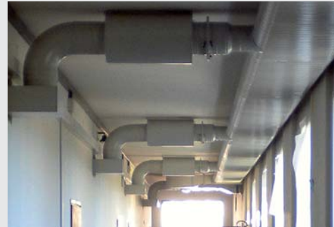
Ventilation ducts at Tito Maccio Plauto School
